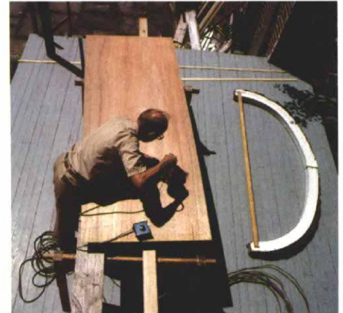
Using an arch detail from the old laundry room as a model, the author cuts out the arch that will fit between columns.
